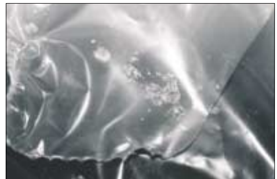
Figure 2: White deposit found on polyethylene packaging wrap also seen on numerous corroded components
