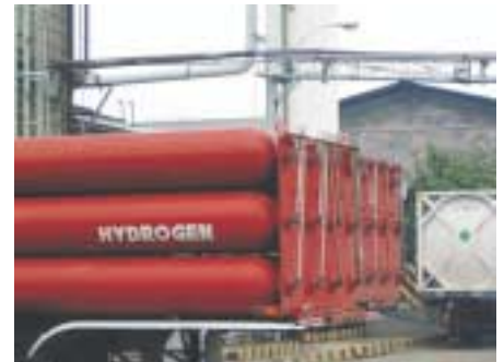
Trailer mounted bank of Hydrogen cylinders
